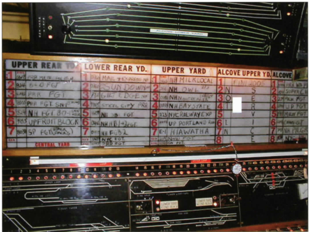
Main dispatching panel and yard assignment board which controls all yards and track switches on the layout.
