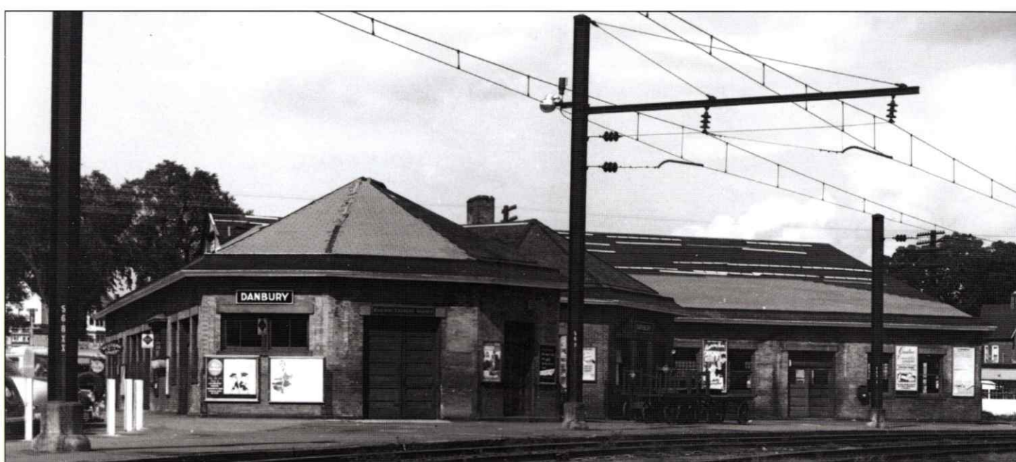
This Charles Gunn photo of the side facing the Norwalk main shows that a roof replacement is in process in August 1954, probably following removal of the last of the platform shed covers earlier in 1954. The double door (the one without glass or transom) facing the photographer is one of two accessing the express room. Photo: NHRHTA Collection
